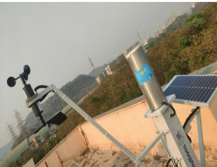
Wind Sensor Boom — Close-up
