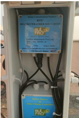
RTU & Charge Controller
